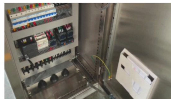
Operator control system
